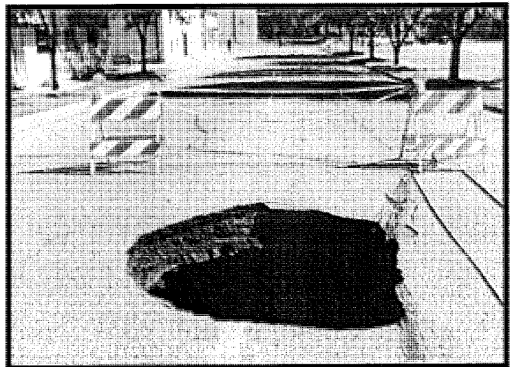
Flood related sinkhole
