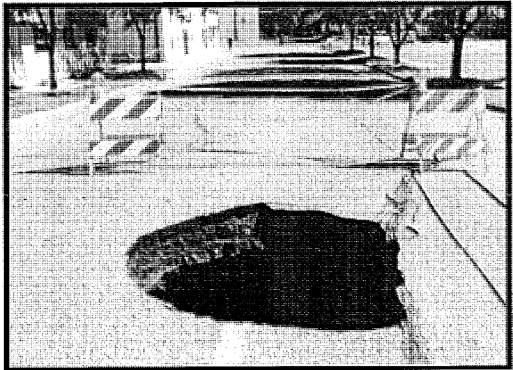
Flood related sinkhole
