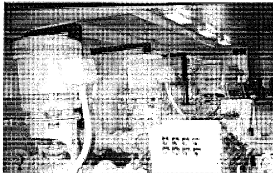
Water treatment plant removes iron and manganese, disinfects and adds fluoride to water supply.
