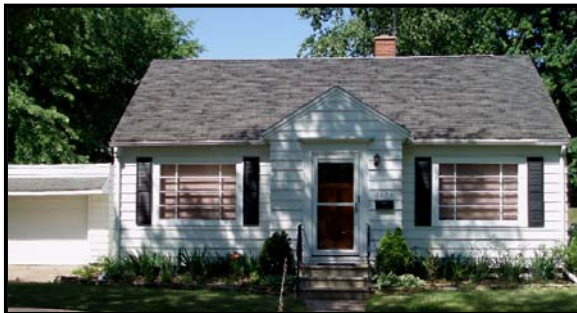
2044 12 th Street – Before Rehabilitation
