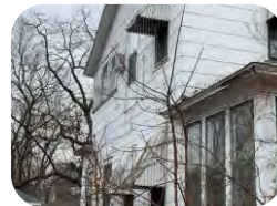
Missing 2 nd exit platform
