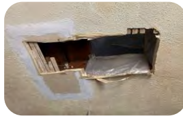
Hole in ceiling from leaking plumbing
