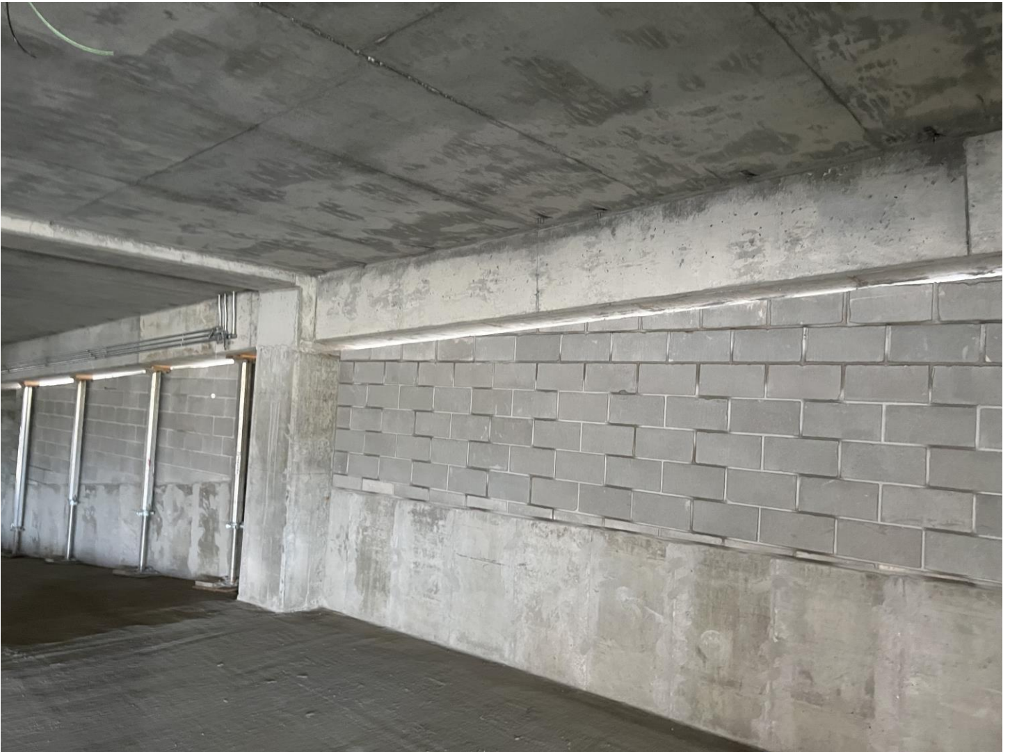
Photo 7 –CMU along Grid E in lower levels. Contractor to install top steel supports per drawings
