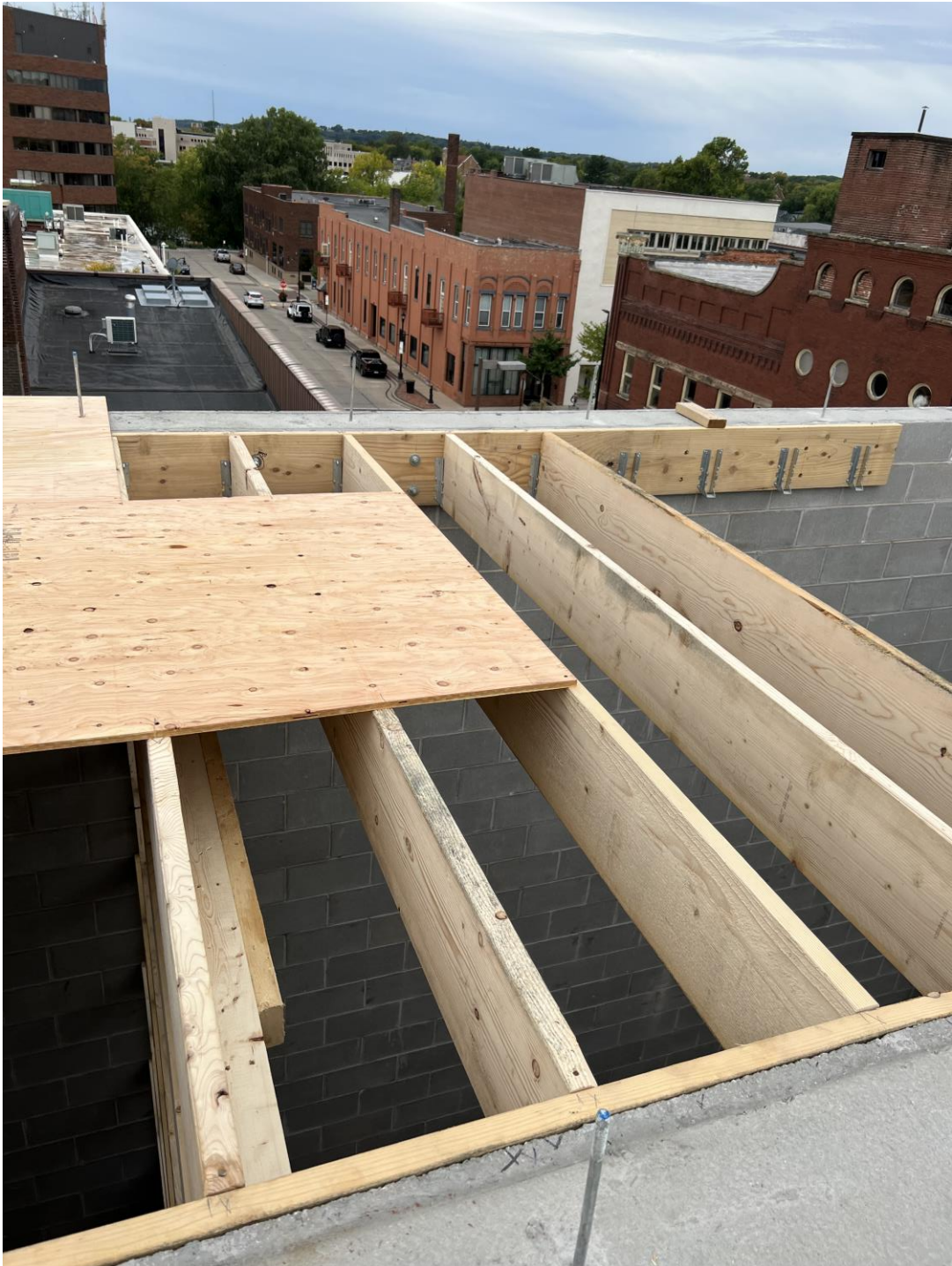
Photo 6 – Wood shaft cover over Stair/elevator core along Grid E. Contractor did not provision wall reinforcing for future expansion as requested in PR 21. This will need to be addressed by the engineer of the future vertical expansion.
