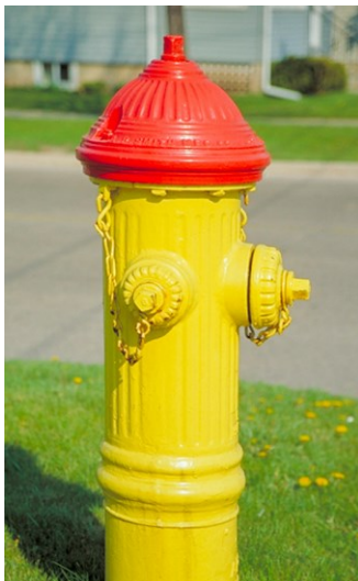
This section of the chapter outlines preliminary plans for extending water and sanitary sewer lines into future service areas,
