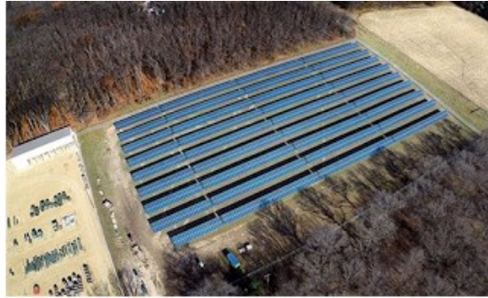
Eau Claire Energy Cooperative's 872 kW Community Solar Array
