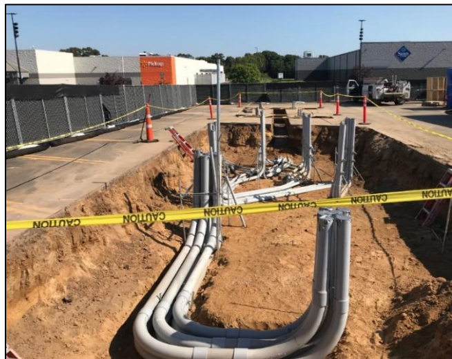
Parking lot retrofit for EV charging stations, Eau Claire, WI (City of Eau Claire)
